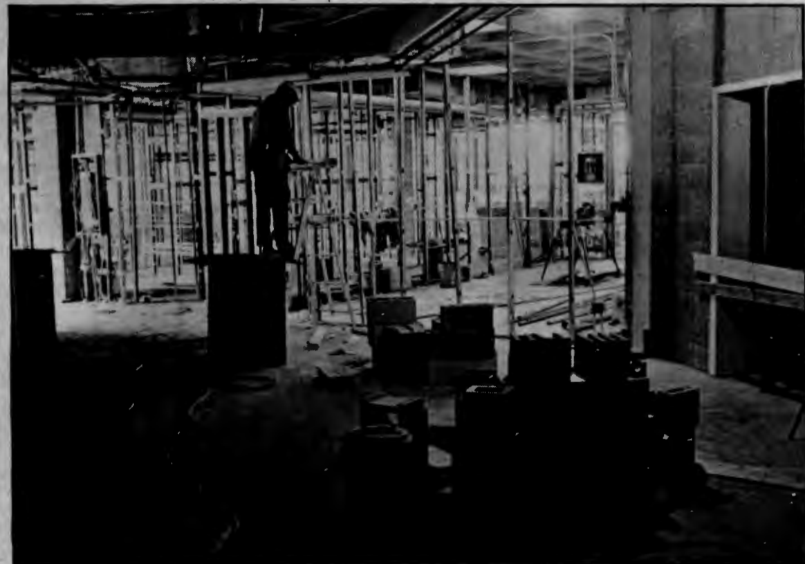
Construction continues on schedule on the Union addition, with the third floor nearing completion. Story page 3.
