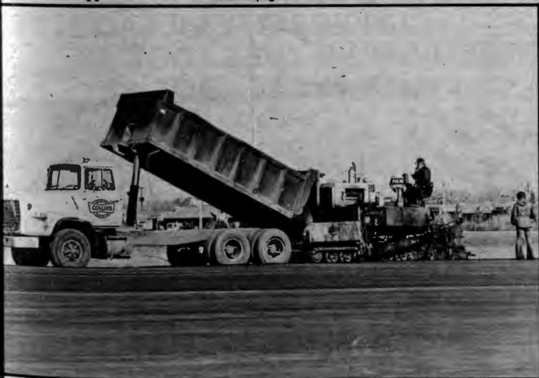
Construction Company is adding a 200 by 500 foot addition to the present parking lot north of the New House. The 330 car addition will bring the total all weather parking space in the lot to over 770 cars. Completion date for the pavement is scheduled for this weekend. (Photo by Matt Caulfield)
