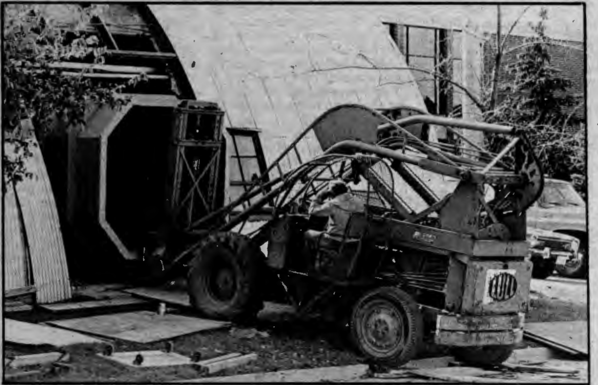
Workers prepare to remove a section of the windtunnel once used by the engineering department. (Photo by Matt Caulfield)
