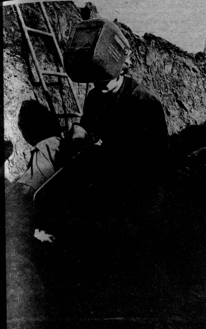
Burkholder Ken Paulus melts a patch over a hole in the steamline that lies in the bottom of the trench north of the Union. It is hoped the patched line will continue sending heat to Churchill and the other buildings along University Drive for a few more years before having to be completely replaced. (Photo by Gary Grinaker)
