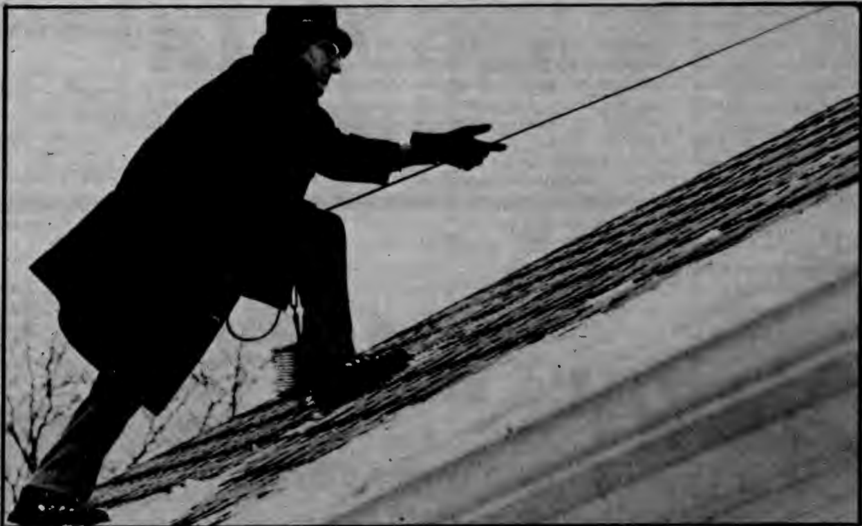
"This is the fun part of the job," Doug said referring to getting up to the chimney to brush it out.
