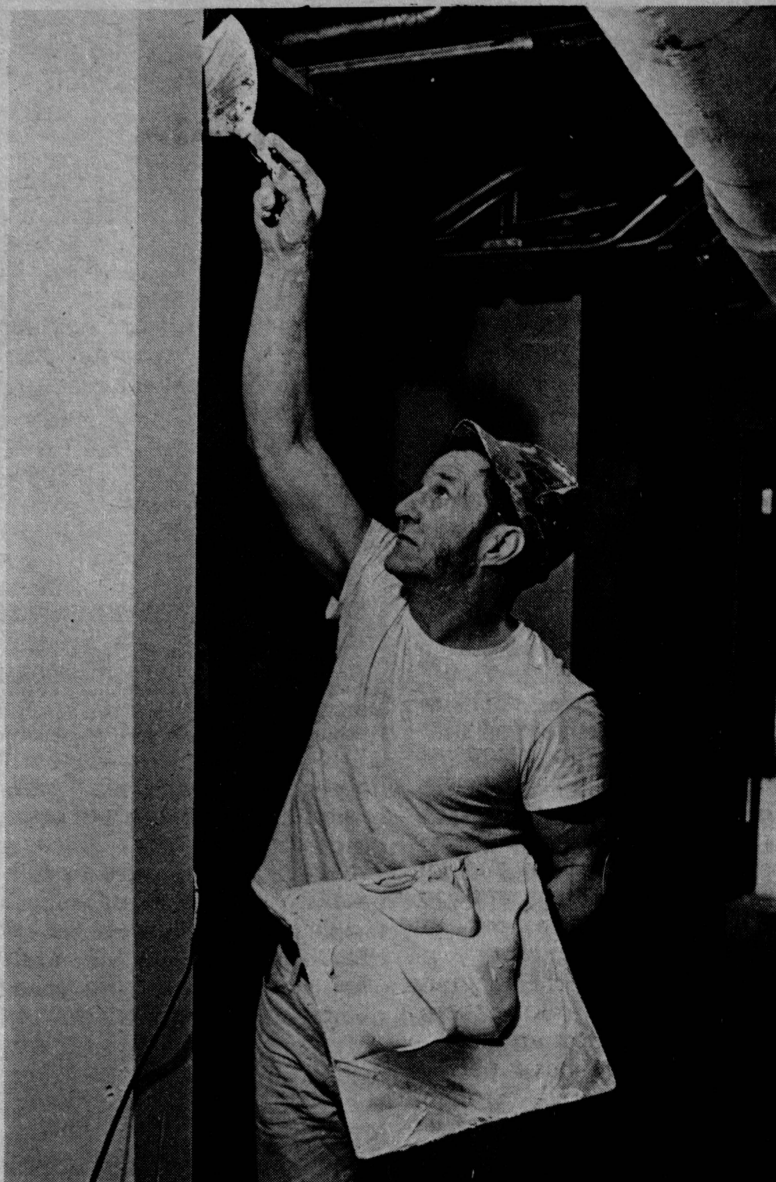
The renovation of the Old Fieldhouse is nearing completion. Roger Hendrickson plasters up a few rough spots in the new locker rooms in the Fieldhouse basement.
