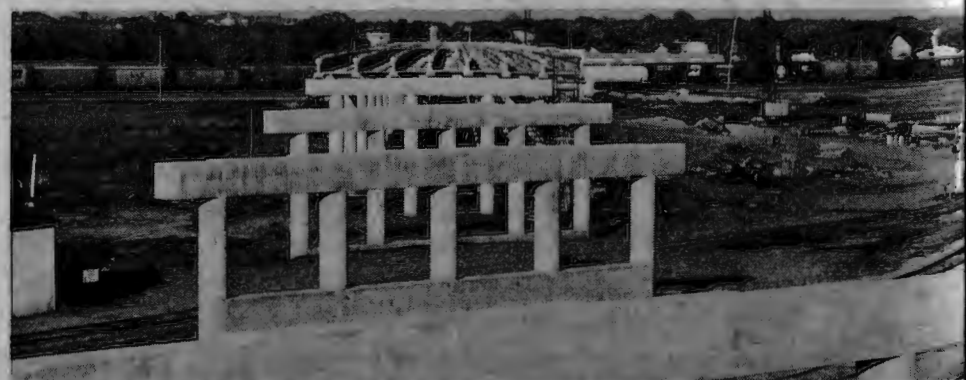
The structural support for the bridge awaits the deck to be laid over the of them
