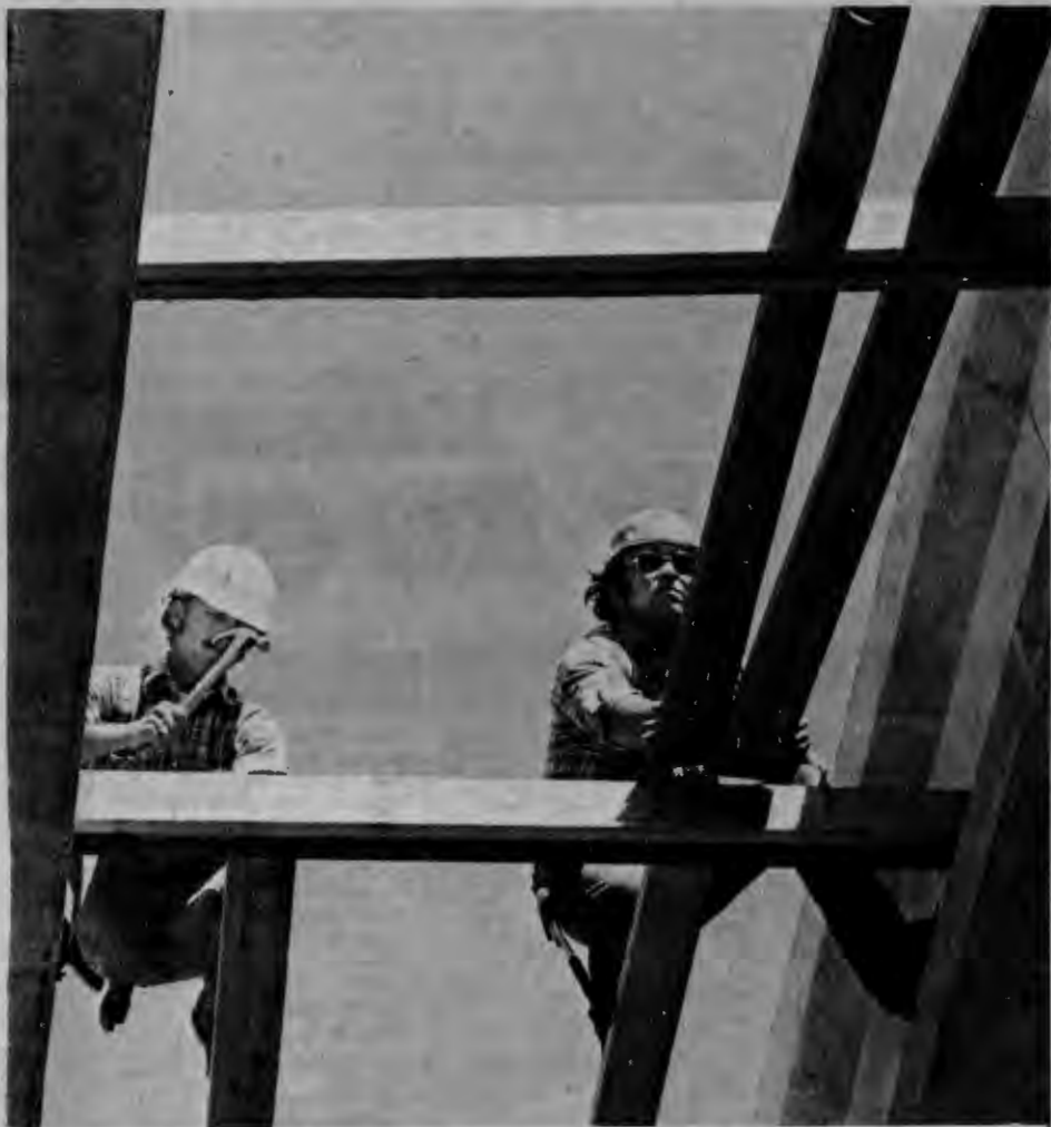
Two of the workers lay down planks that will eventually be covered by cement.
