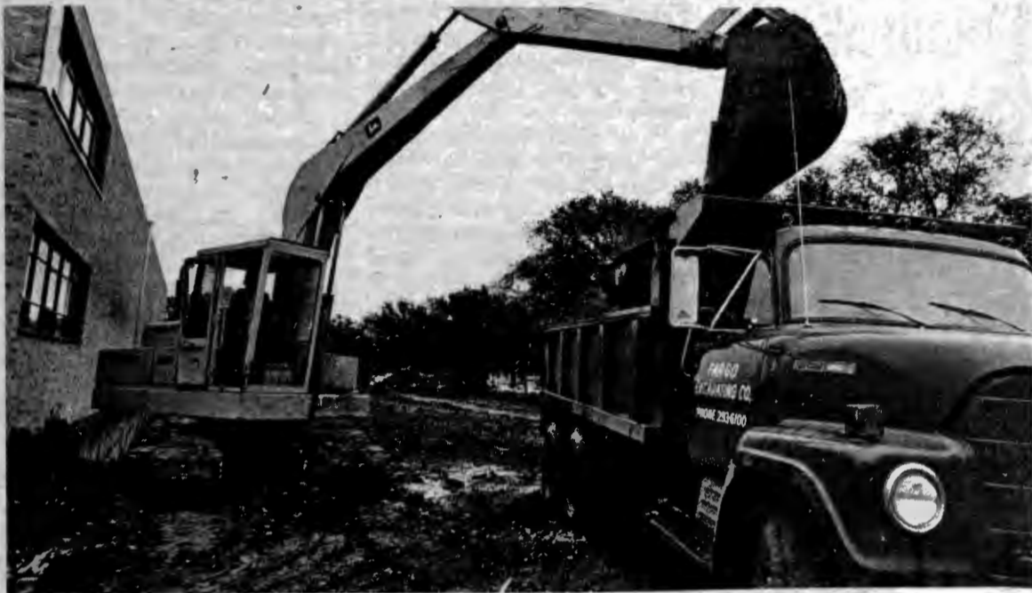
In spite of the rain and mud, construction on the new library addition started Tuesday. (photo by Gary Grinaker)
