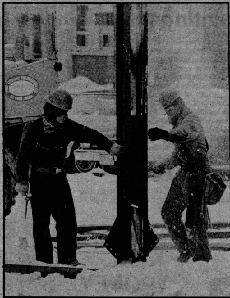
One of the workers gets doused with some of the snow that he was knocking off the steel beam.
