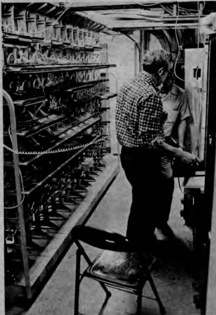
Northwestern Bell employees install SU's new phone system that will become operational March 5. (Photo by Don Pearso)
