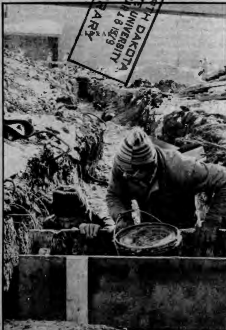
Butch Puhalla and Ed Cegla of Midwest Mechanical Contractors work on a concrete anchor for the supplemental steam line to the library to service the new addition (Photo by Andre Stephenson)
