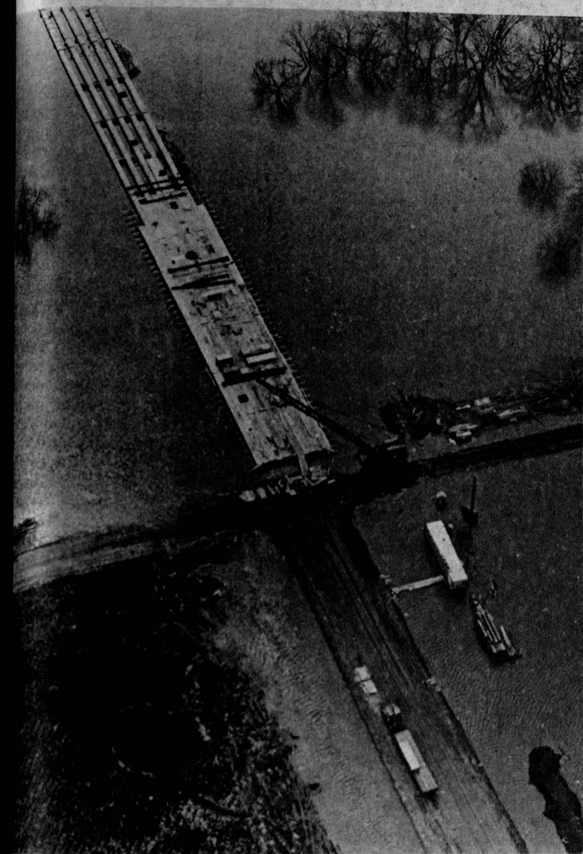
A crane was brought in to raise a road north of Fargo so the traffic can continue moving over it.
