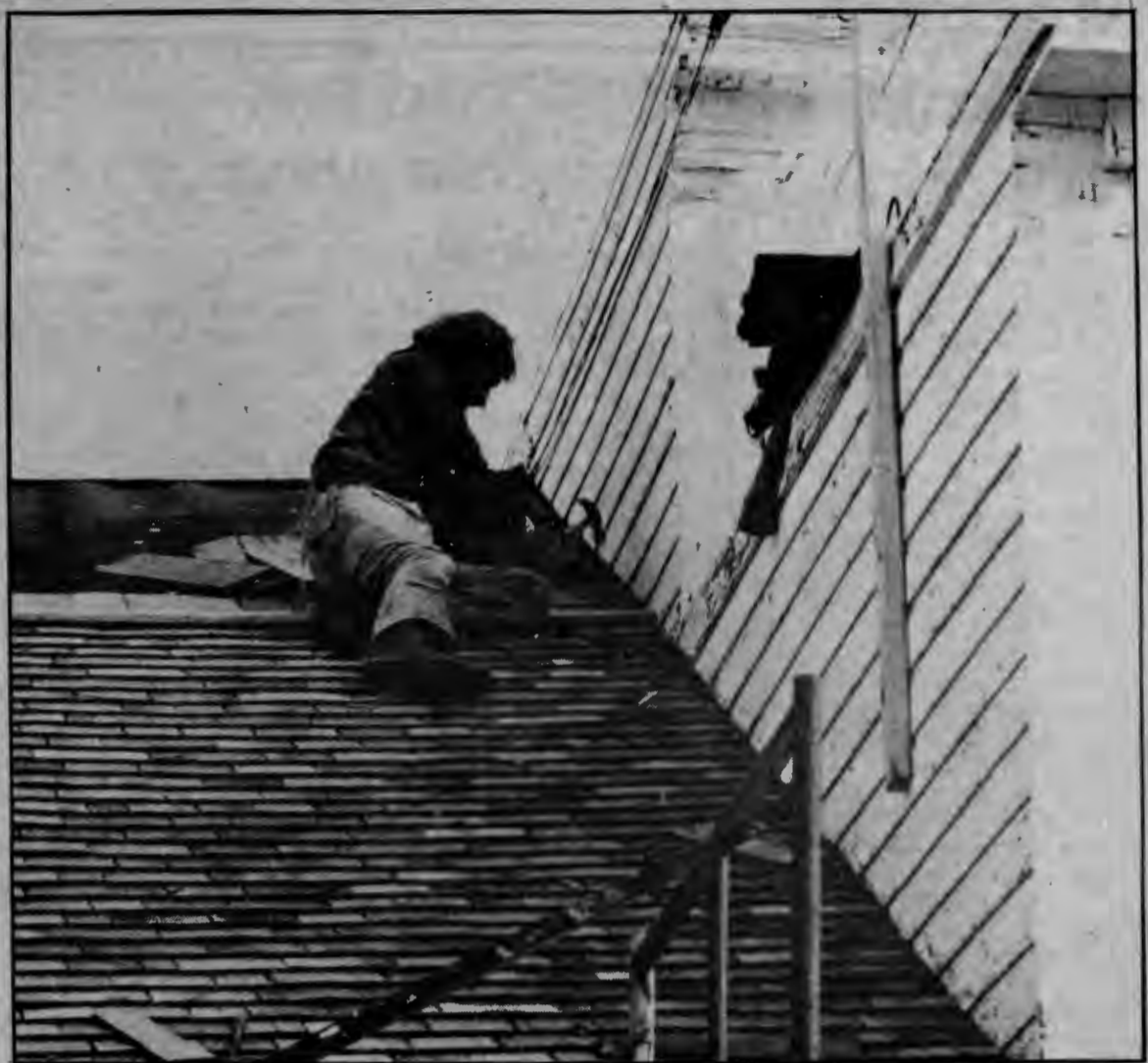
Workers attempt to patch the holes in the roof on Festival Hall.
