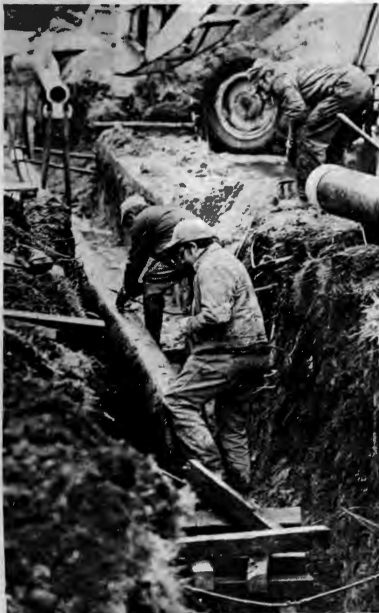
Yes, Virginia, there is a West College Street. Construction and rejuvenation on SU's most pleasant route continues well after estimated dates of completion, but relief may be in sight. Traffic is expected to begin moving through WCS in late September.
