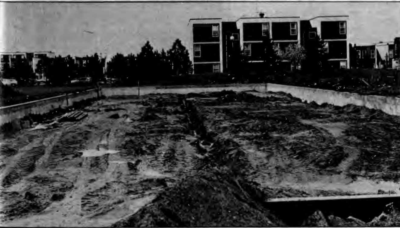
Construction on another unit of married-student housing is underway on the north edge of University Village. When completed 17 more apartments will be available for married students. The building is slated for completion in time for occupation fall quarter.
