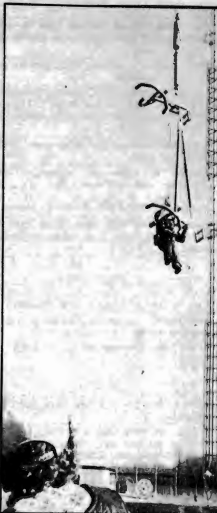
Darrel Biteler (in cap) and Wayne Resel of a local tower service lift two elements of SU's new broadcast antenna to the top of the tower near Amenia, N.D.
