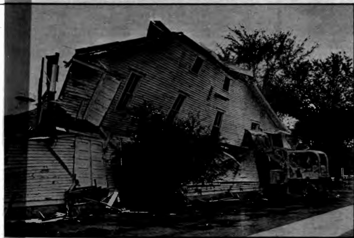
Last wall of Festival Hall was the last wall to fall under the push of a bulldozer.
