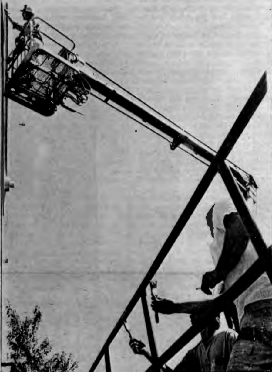
Buildings and grounds personnel painted railings and windowsills on Dinan Hall Tuesday with the aid of a moveable boom mounted on a truck.
