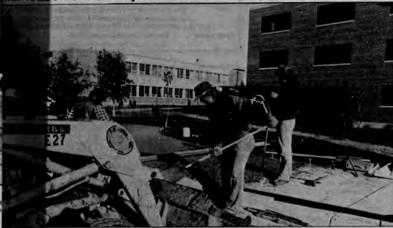
Workers from F-M Asphalt Company put some finishing touches on the new parking lot where Festival Hall once sat. Asphalt paving was installed after this photo was taken.
