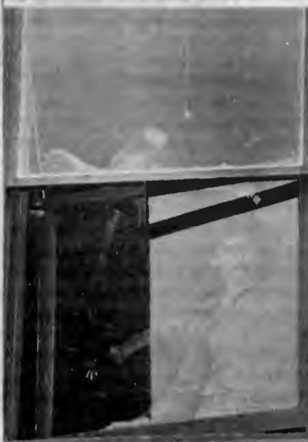
Arlie Trangsurd and Allan Cossette install a new window in South Engineering. By the way, it was Friday the 13th.
