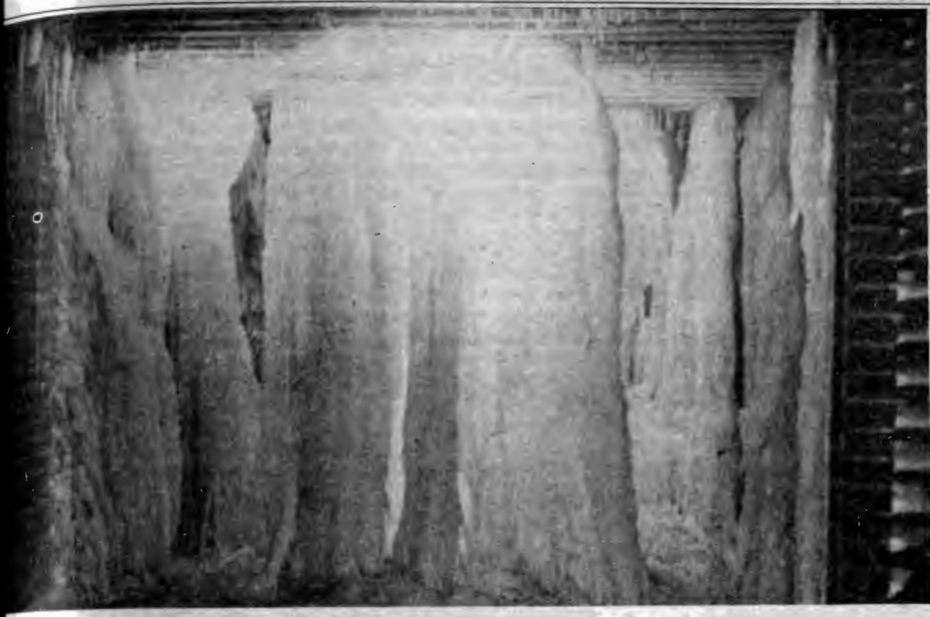
Ice formations appeared in the tunnel underneath the FLC building. The ice was formed when water pipes broke during the rigid weather over the Christmas holiday. (Photo by Badea Rashedy)
