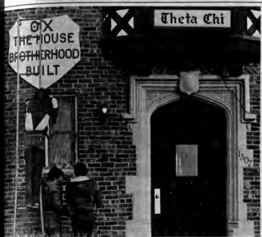
The Theta Chi house was built with brotherhood. But the winter weatherizing was done by Brett Loftesnes, on the ladder, Chris Bartsch, center, and Dale Ekheimer, right, Tuesday afternoon. (Photo by Bob Nelson)
