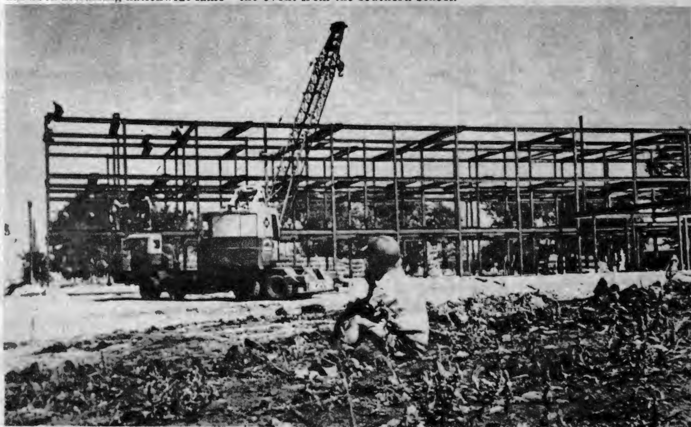
The construction of Burgum Hall was one of the major building projects on campus in 1961.
