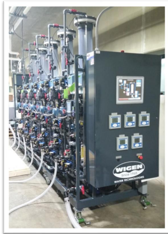
Figure A1: Photograph of Filter Pilot Skid Located Within MWTP
