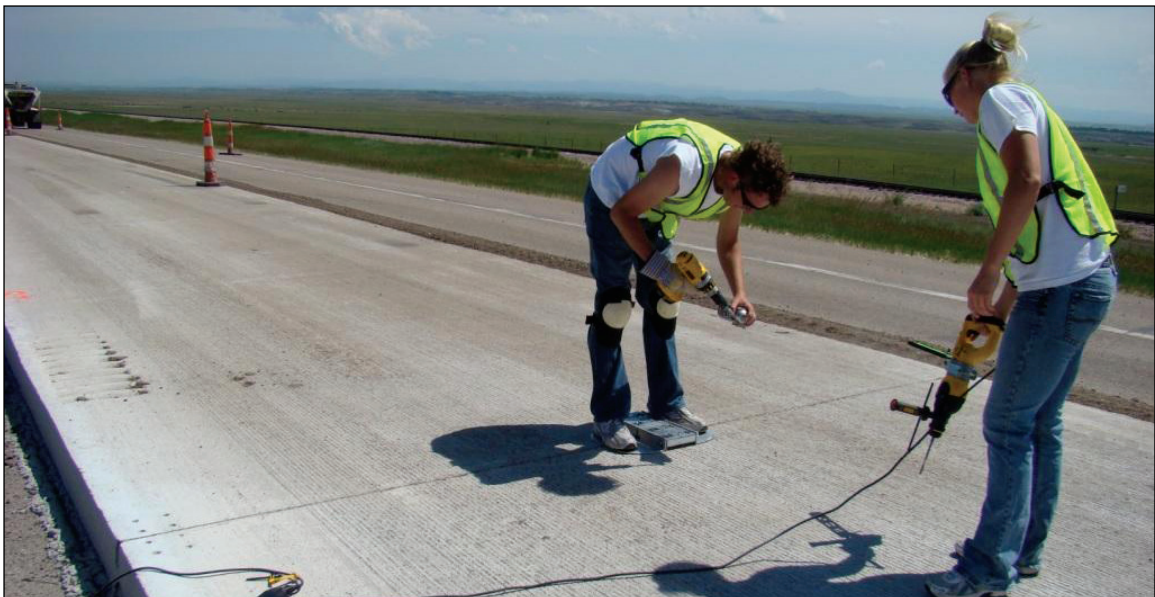
SDSU graduate students installing joint instrumentation on U.S. Highway 212 west of Belle Fourche, SD.
