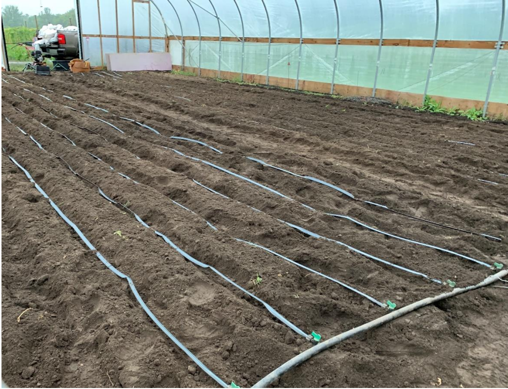
Figure B6. Drip tape installation after rototilling in high tunnel near Absaraka, ND.
