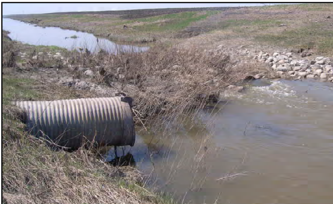
Picture 9 - Rock and culvert structure on the Rush River within the study area. Photo from April 22, 2010.
