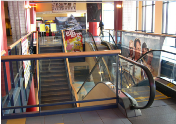
Figure: B-52 Crown Block E Escalators
