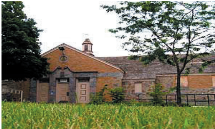
This is the South elevation of the pool building. It is currently not in use. This building is located on the South West end of the site.
