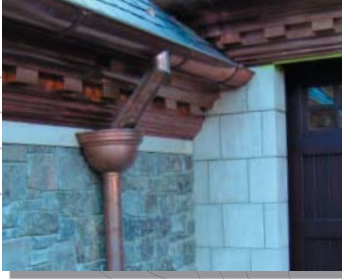
Metalwork Style To be used.
