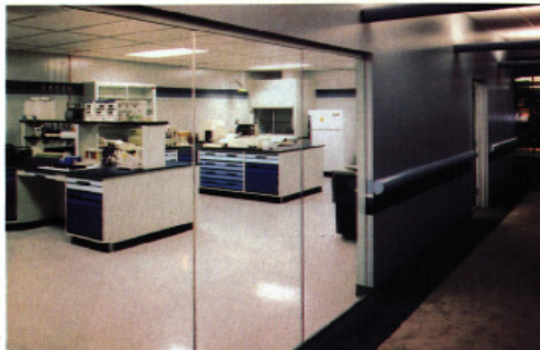
Below, flexible HVAC system of the Serono DNA lab allows a wide variety of lab types. Note observation corridor.
