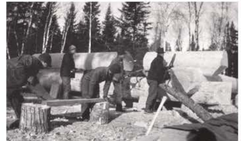
Figure 2.3. The Old Timer's Cabin was the first building constructed by the CCC in Itasca State Park in 1934
