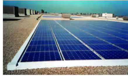
Photovoltaic Roof Panels
