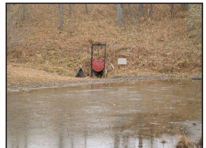
Control of the Land - Fall 2005 Control culvert - south end of the site
