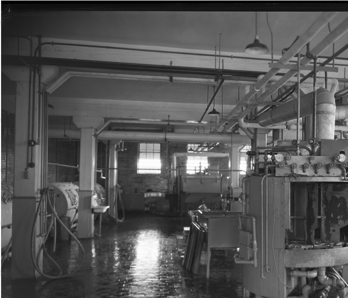
Refrigeration Plant in the basement, 1930's.
