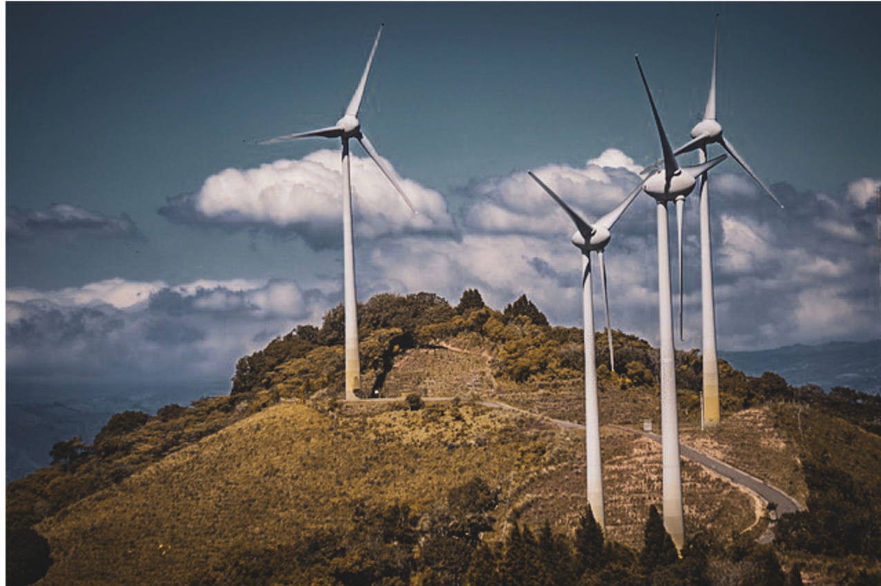
GUANACASTE WIND POWER PLANT
