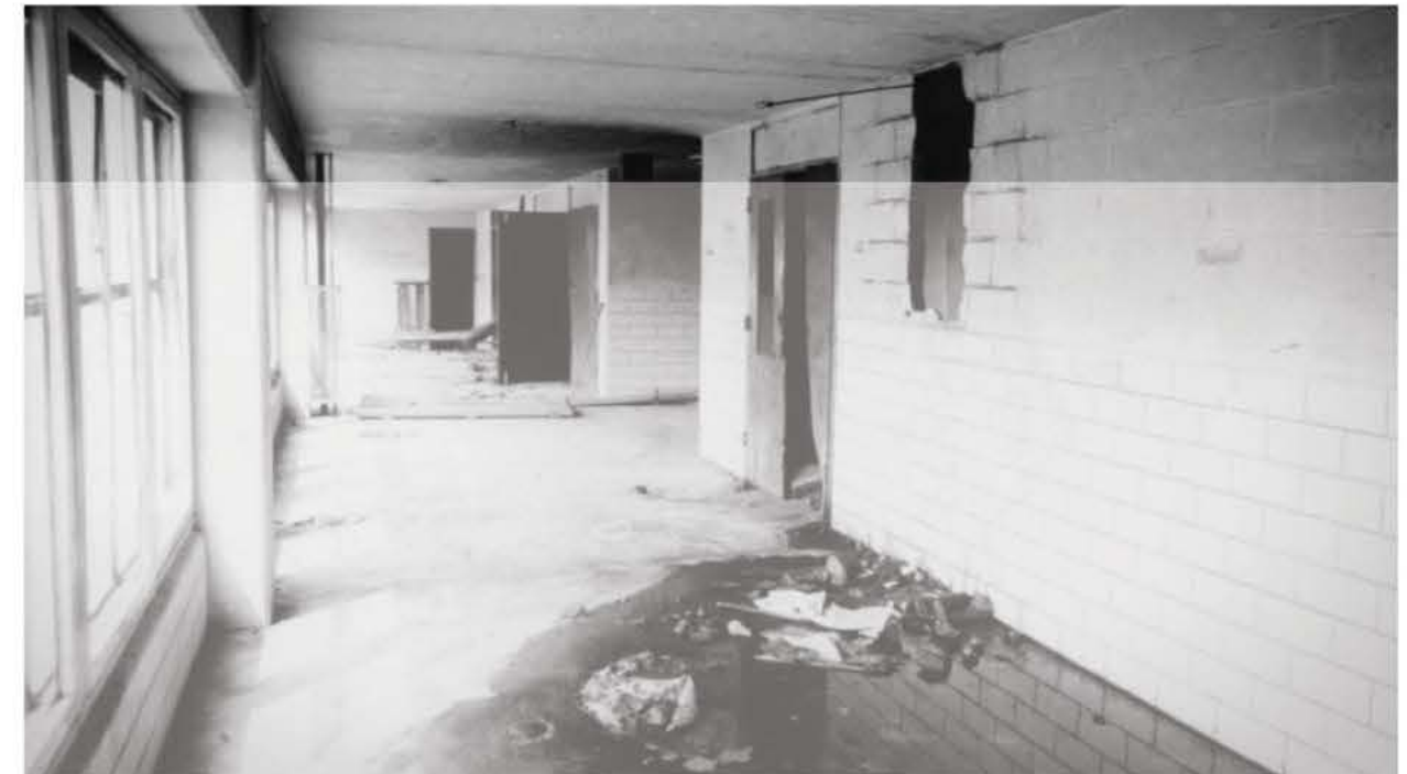
Fig. 018 | Decayed Gallery | The Pruitt-Igoe Myth
