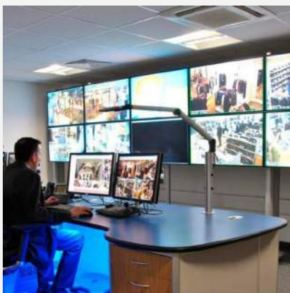
Figure 172—CCTV Control Room (from Evolution News)
