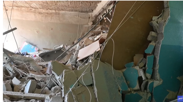
COLLAPSED INTERIOR WALLS
