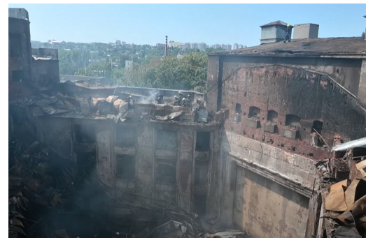
AUDITORIUM AFTER SHELLING
