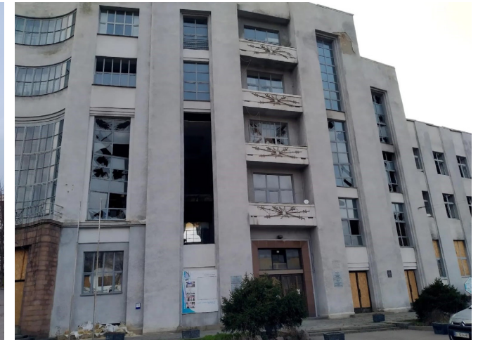
EAST ENTRANCE AFTER SHELLING SHOWING BLOWN OUT WINDOWS
