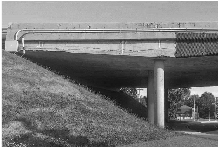
Figure 1. A bridge with serious damages ( https://www.fprimec.com/testing-damaged-bridges/ ).
