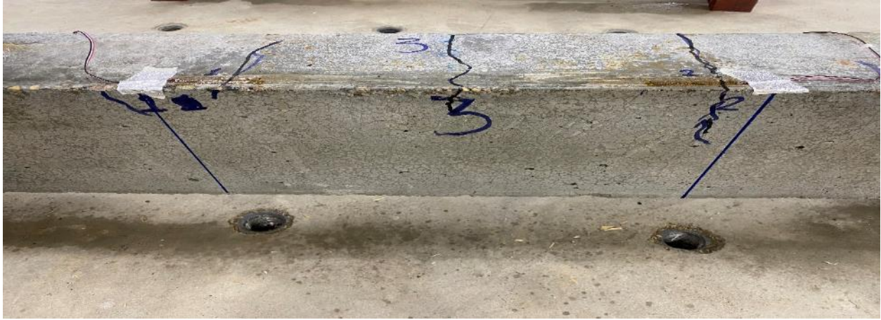
Figure 46. Cracks for Sample 3 after the Test
