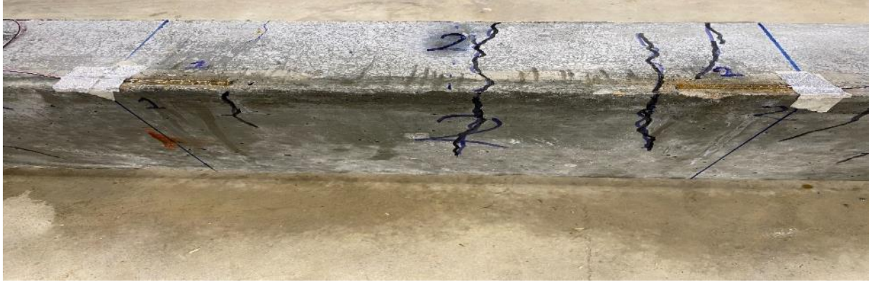
Figure 40. Cracks for Sample 2 after the Test
