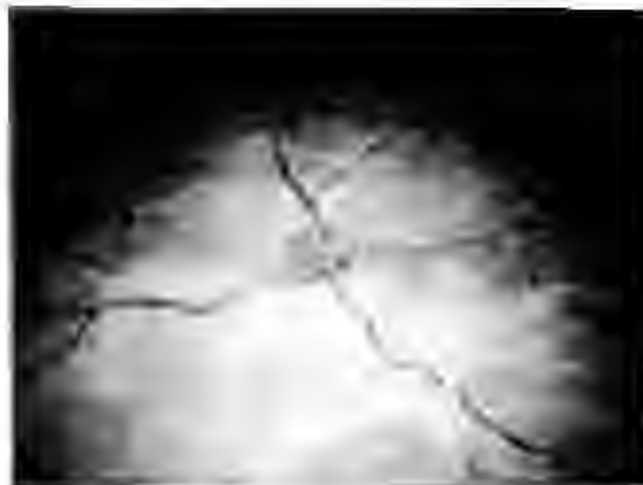
Figure 2.2. Example of concrete cracking from freeze-thaw effects (McDonnell 2007)
