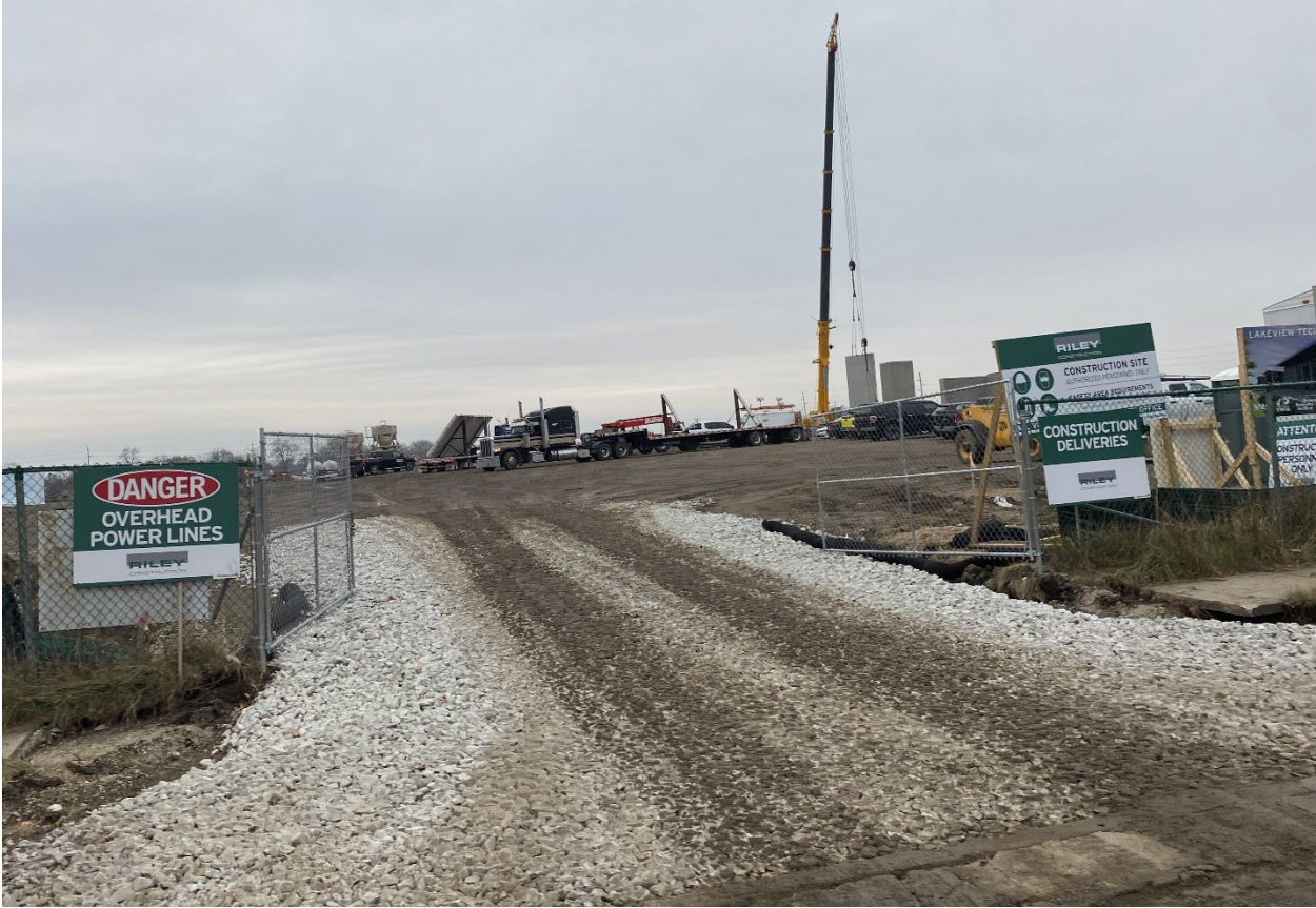
Figure 9: Site Photograph (December 2023) This site photo facing south shows Lakeview Technology Academy being built.
