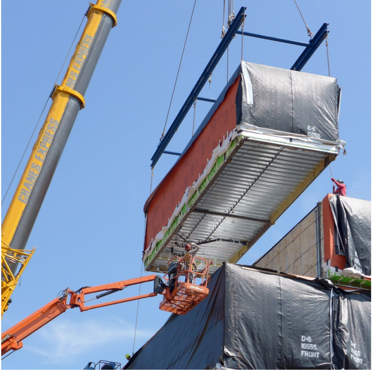
Figure 50. Picture of a module being lifted into place to be secured to The Stack. Credit: GLUCK+
