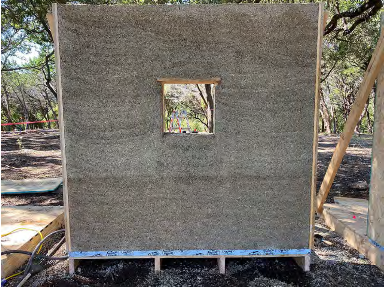
Figure 45. Frame on Center Hempcrete Wall Construction Note: Hempitecture. (2020, May 5). Hempcrete Wall Detailing. Hempitecture Inc. https://www.hempitecture.com/post/hempcrete-wall-detailing
