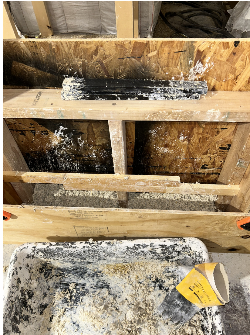
Pack the mix into the wall using slip forms and a stick to pack the mix tightly into corners.
