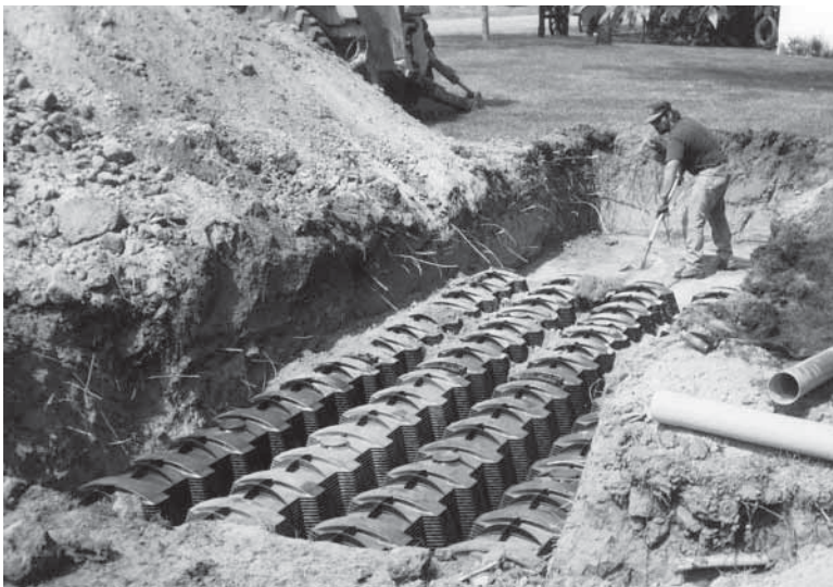
Figure 17. Chamber-type gravelless system being installed on a very small house lot. Normally the chambers would be used in trenches.
