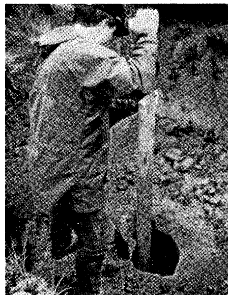
Tamping native clay as it is shoveled into the well is an important step to insure that all voids are filled and minimal settling will occur.
