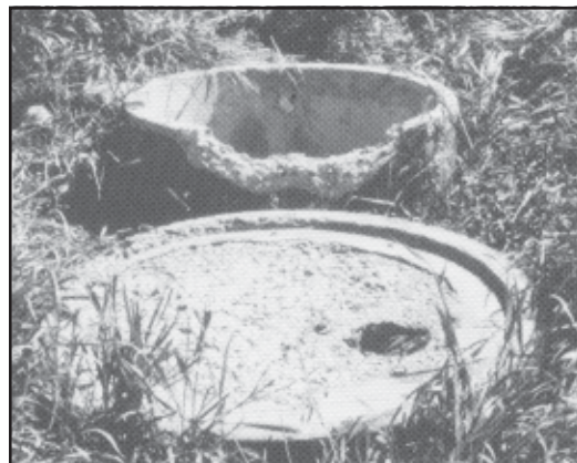
Initial well-plugging steps include accurate measurement of the well dimensions and removal of all obstructions.
