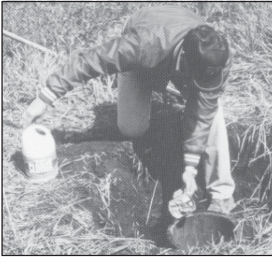
The chlorination procedure disinfects the well so that disease-causing microorganisms are not sealed in the aquifer after the well is plugged.
