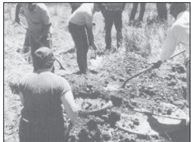
Abandoned wells with diameters of 10 inches or greater are usually plugged with a combination of materials such as sand gravel and native clay. These materials should always be shoveled into the well, as opposed to being dumped rapidly in large quantities.
