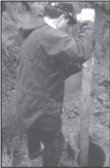
Tamping native clay as it is shoveled into the well is an important step to insure that all voids are filled and minimal settling will occur.
