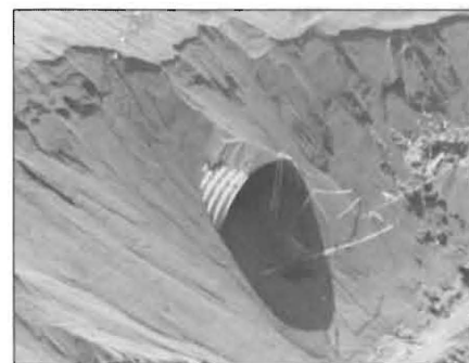
Figure 1. Sediment displaced by wind erosion events fill road and drainage ditches, impede water flow and may impact water quality.
