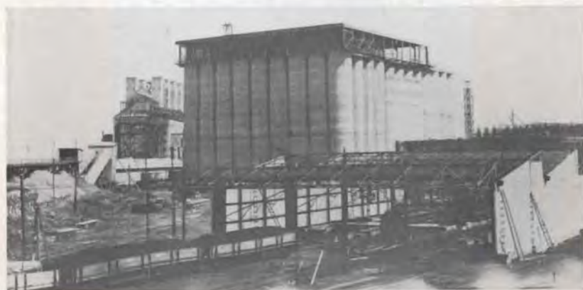
This elevator under construction at Bahia Blanca—when finished, will be one of the largest in the world.
